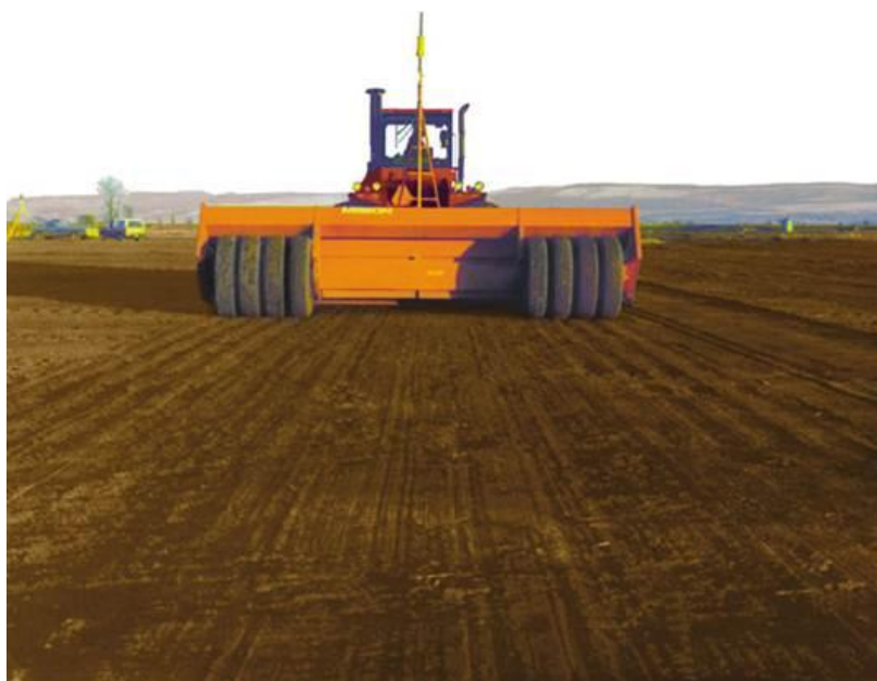
A ripper attachment loosens the ground in the outer area so that field will settle uniformly and settle evenly
